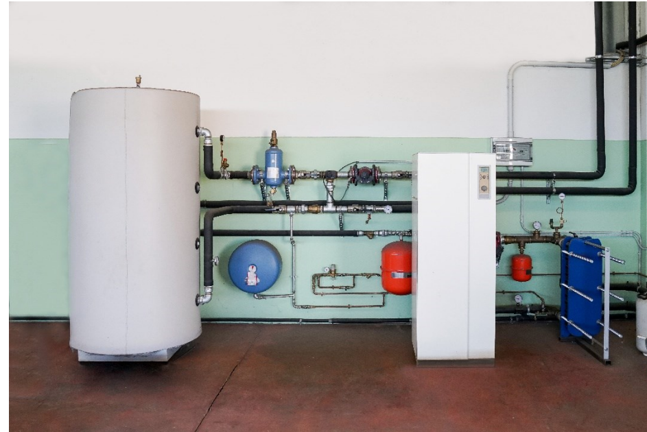
Indoor heat pump and tanks
